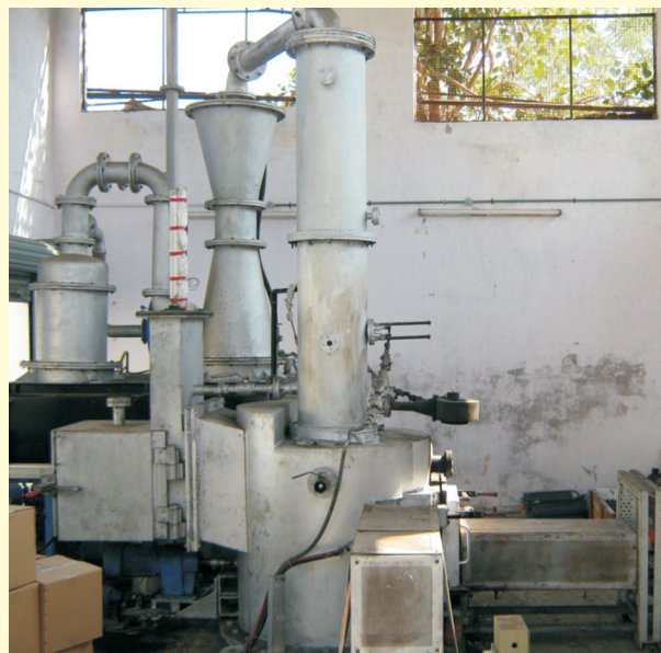
Fig.1: Photograph of the Plasma Pyrolysis System installed at GCRI, Ahmedabad
