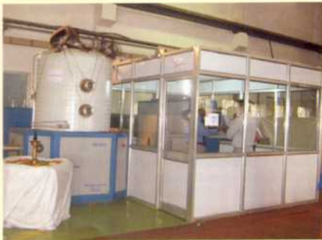
Fig. 1: Photograph of the plasma nitriding system installed at IGTR, Ahmedabad
